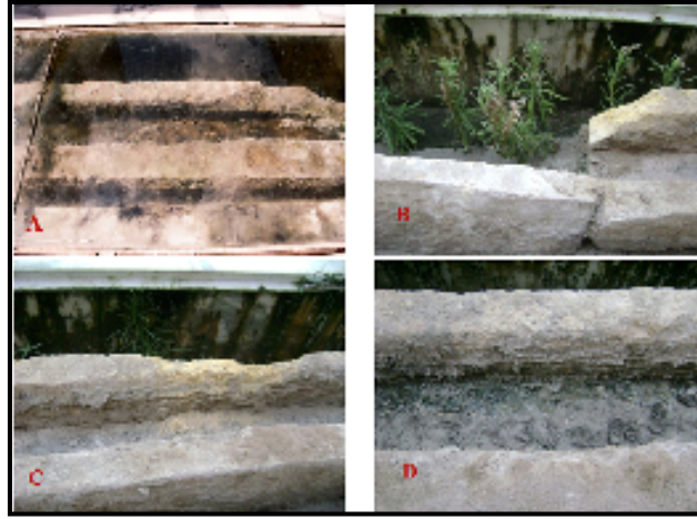
Fig. 4 Shows the degradation phenomena of the water duct. (A) Shows the discoloration of stone surface due to the accumulations of colored stains of microorganisms. (B) Shows the vascular plants growing in the bottom of the water duct. (C) Shows the eroded edges of the water duct due to the exfoliation and detachment of the superficial layer. (D) Show the black crust accumulated on the stone surface
